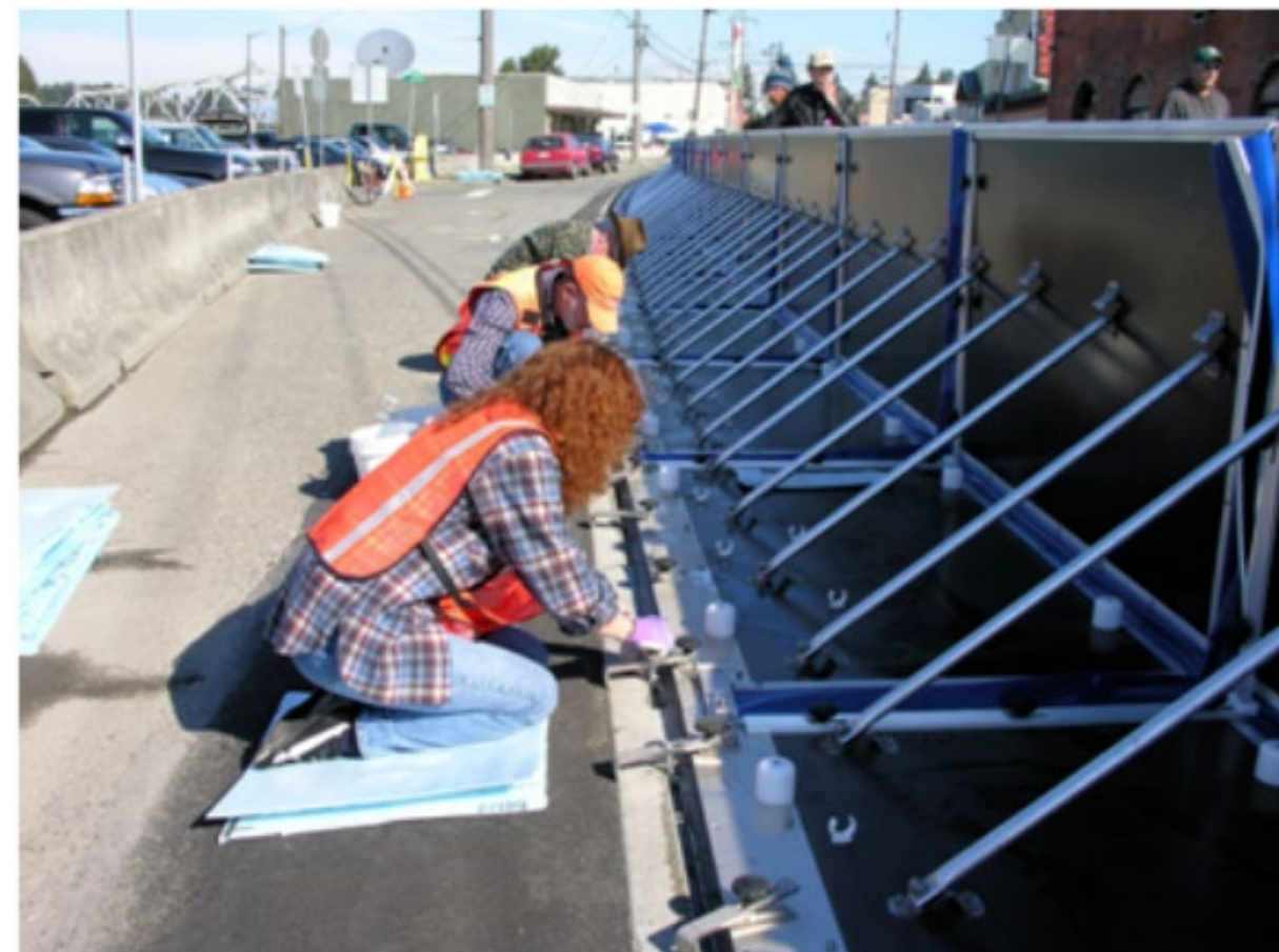
Temporary flood barriers can be effective at preventing flood damage Source: Sustainable Buildings Initiative. Climate Resilience Toolkit.
