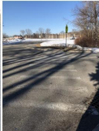
Faded crosswalk at access road entrance to school property
